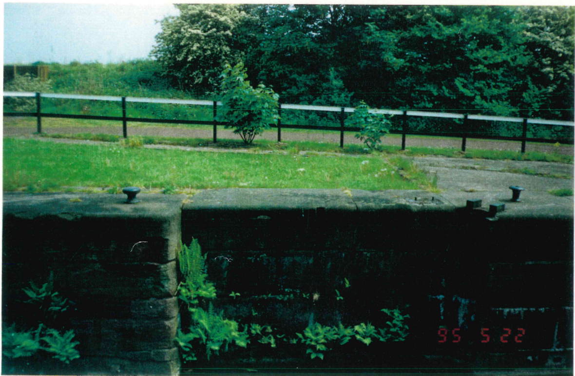
PHOTOGRAPH 3/17 - Downstream Gate Quoin and Missing Gate
