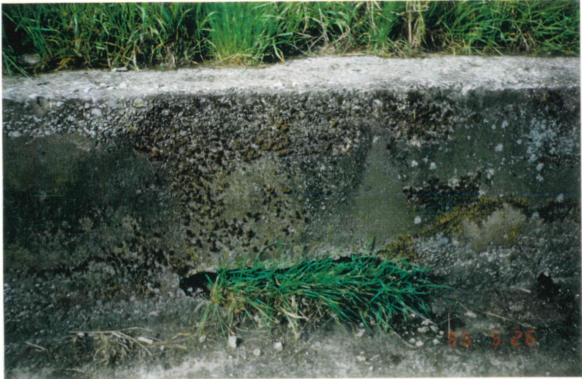
PHOTOGRAPH 6/2 - Void in Concrete Channel Wall
